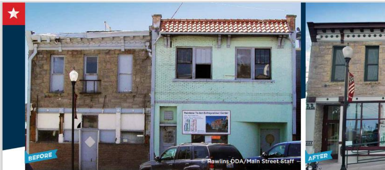
Using a $1.8 million state grant, Rawlins DDA/Main Street restored two dilapidated buildings (above left), one of which was in such a state of disrepair it had been nicknamed the “pigeon hotel.” Today the buildings house the Rainbow Te-ton Entrepreneur Center (above right), which serves as a business incubator, a networking site for downtown merchants, and a community meeting space.
